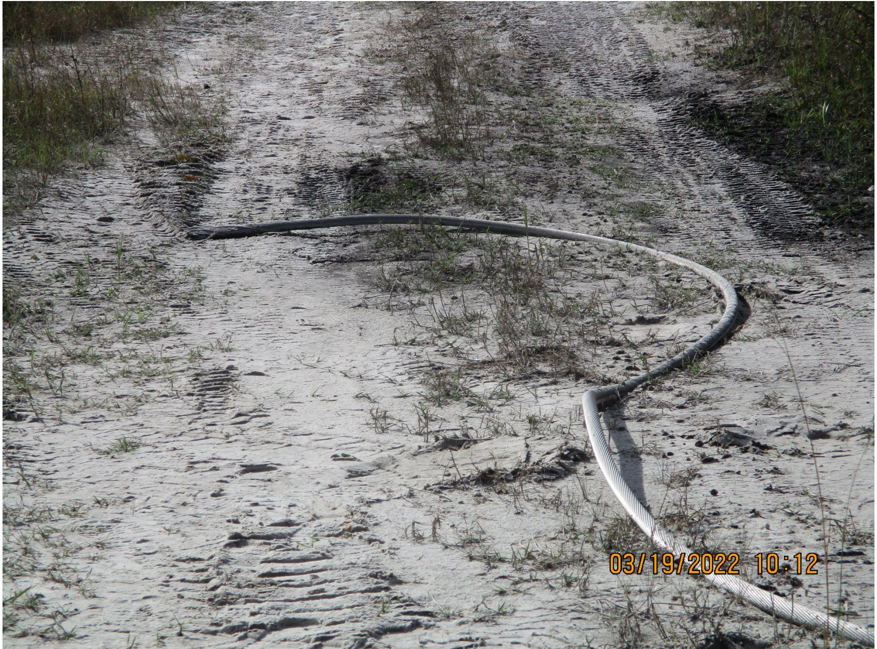
Photo 8 – High voltage power line cut, laying on ground
