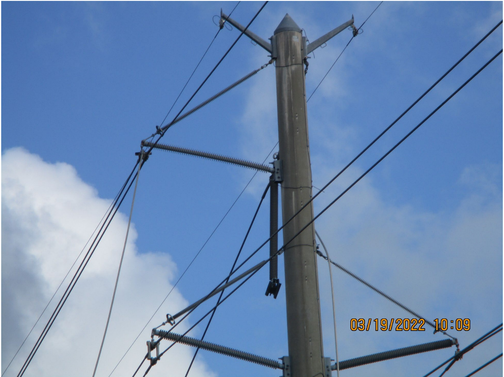
Photo 9 – high voltage power lines cut and broken
