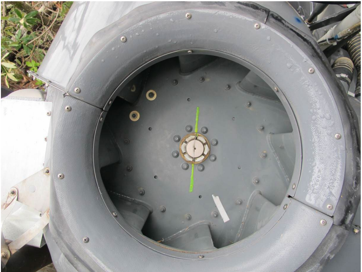
Cooling fan and scroll.
