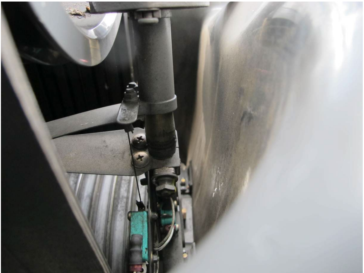
Overtravel switch activation cable.
