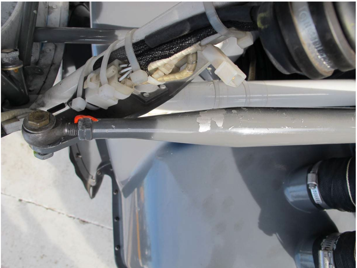
Aft end of C121-15 push pull tube.
