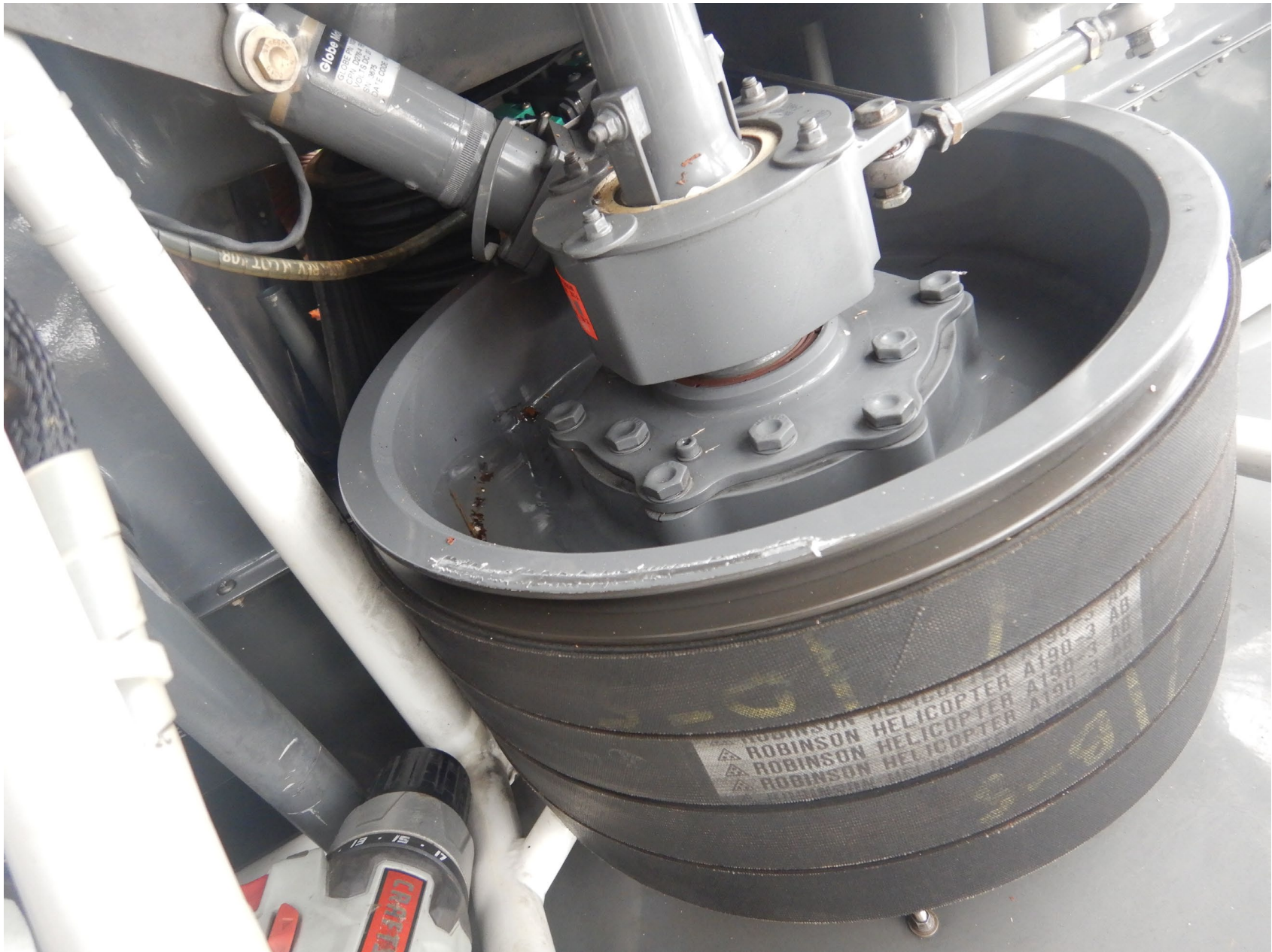
Photo 12 – V-Belts on Upper Sheave (NTSB Photo)
