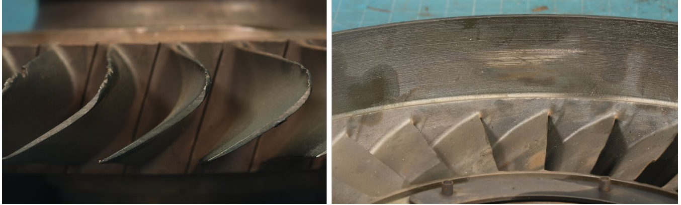
Photo 23- 3 rd Stage Turbine Blade Tip Rub (L), 3 rd Stage Shroud Rub (R)
