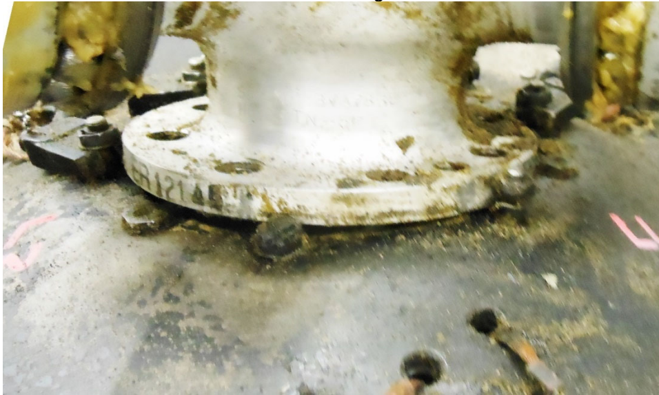
Photo #22 - Fractured/missing start lock brackets
