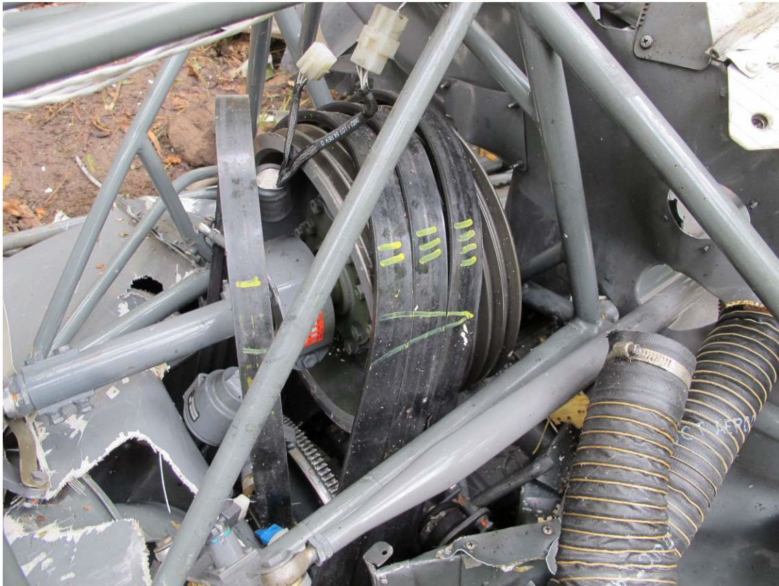
Figure 28 - V-Belts on Upper Sheave
