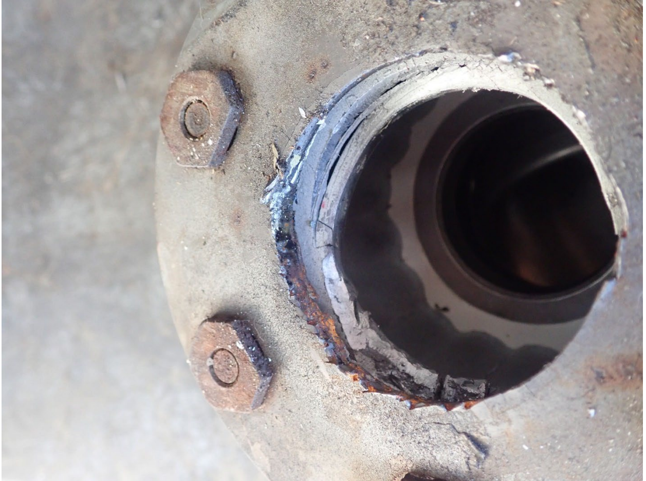
Figure 18 - Propeller Flange Fracture
