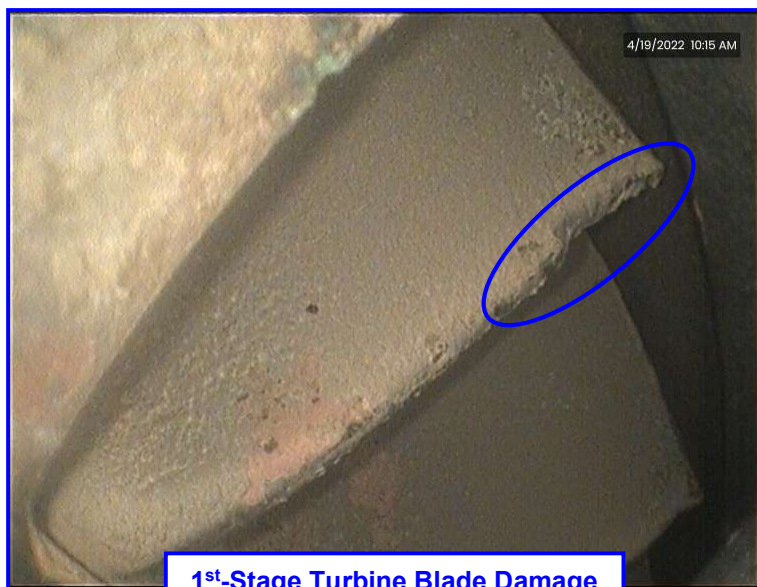
1 st -Stage Turbine Blade Damage
