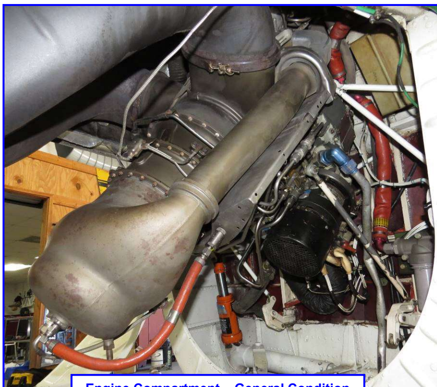
Engine Compartment – General Condition
