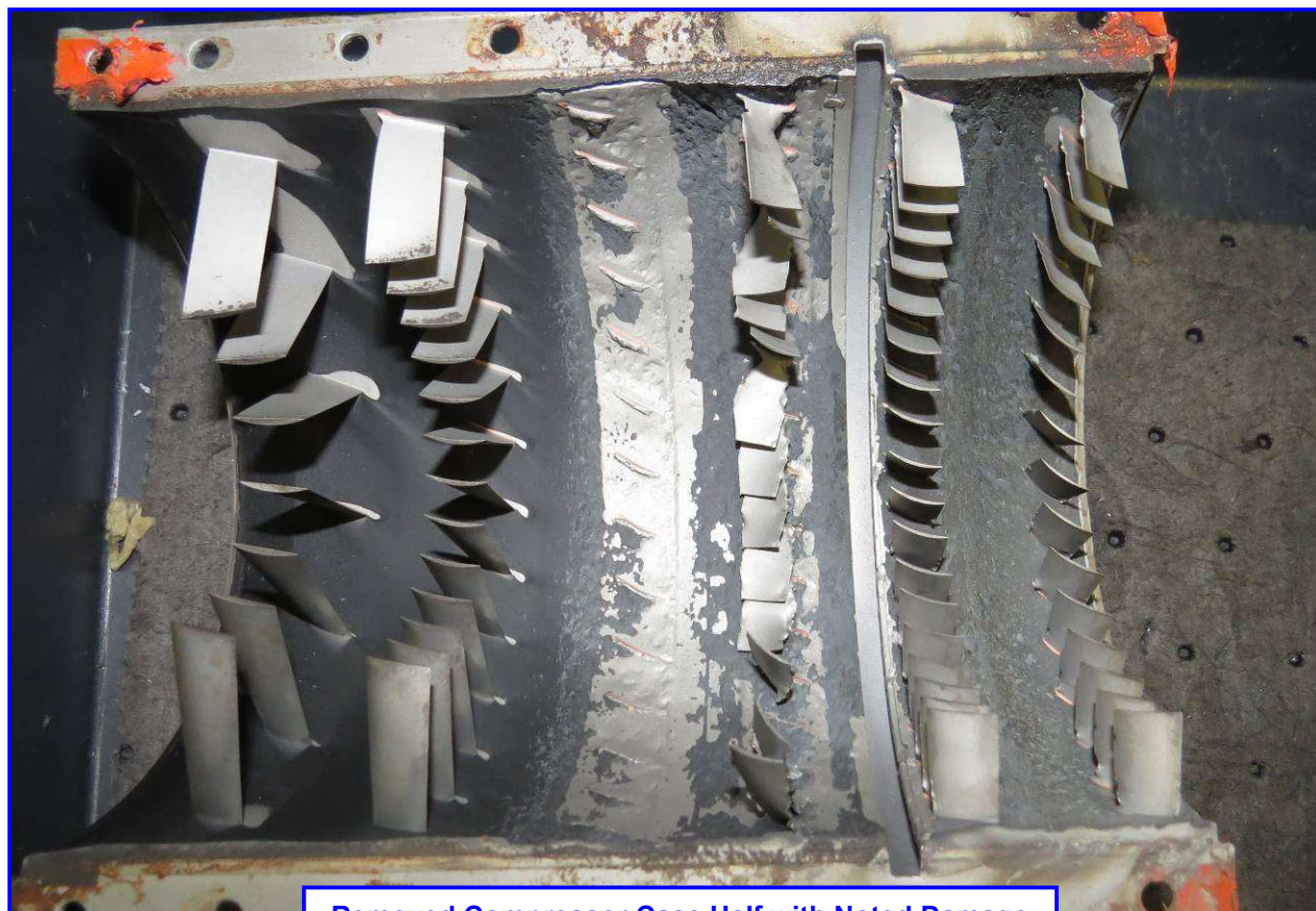
Removed Compressor Case Half with Noted Damage
