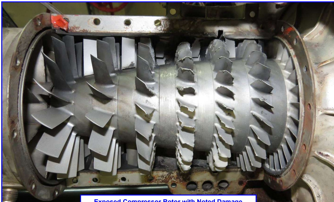
Exposed Compressor Rotor with Noted Damage
