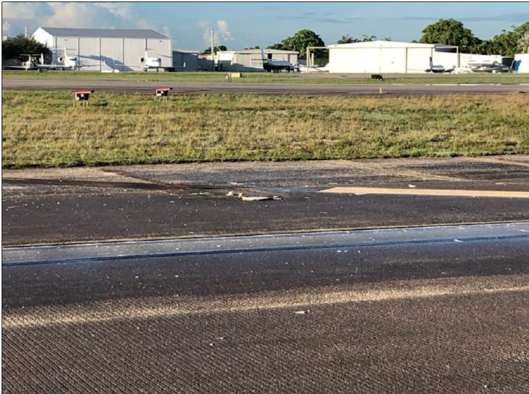
Photo 4 – View of the debris found on the runway after taxiway sign impact (Photo Courtesy of Airport Authority)
