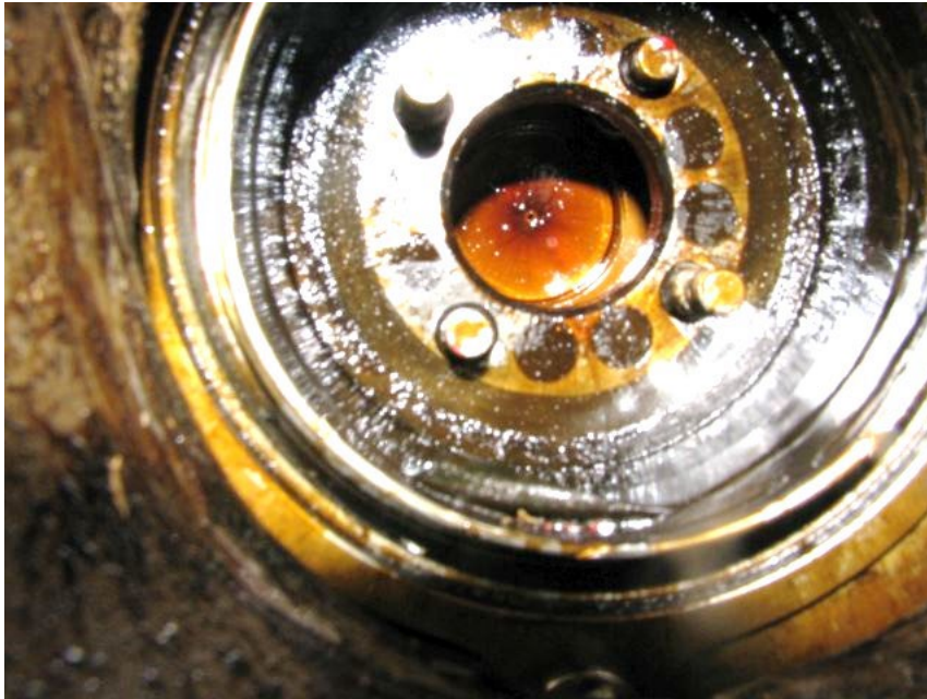
Figure 5 - Main driveshaft inner coupling remained in engine end (courtesy Bell)
