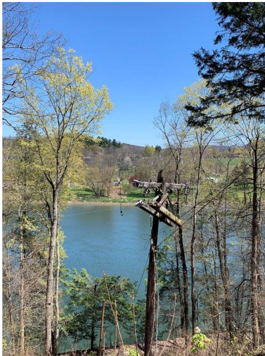
Photo 7 – View of damaged transmission pole/wires. (Courtesy of First Energy)
