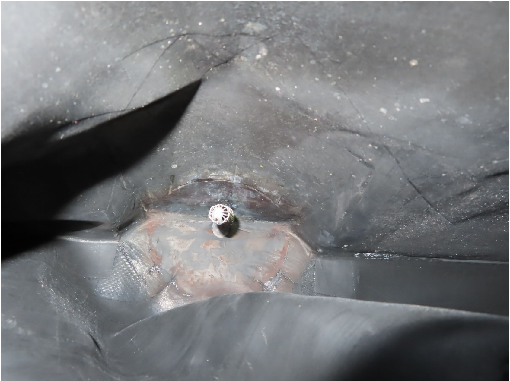
Photo 11 – Right Wing Inboard Fuel Pick-up with Inlet Screen Installed (Piper)
