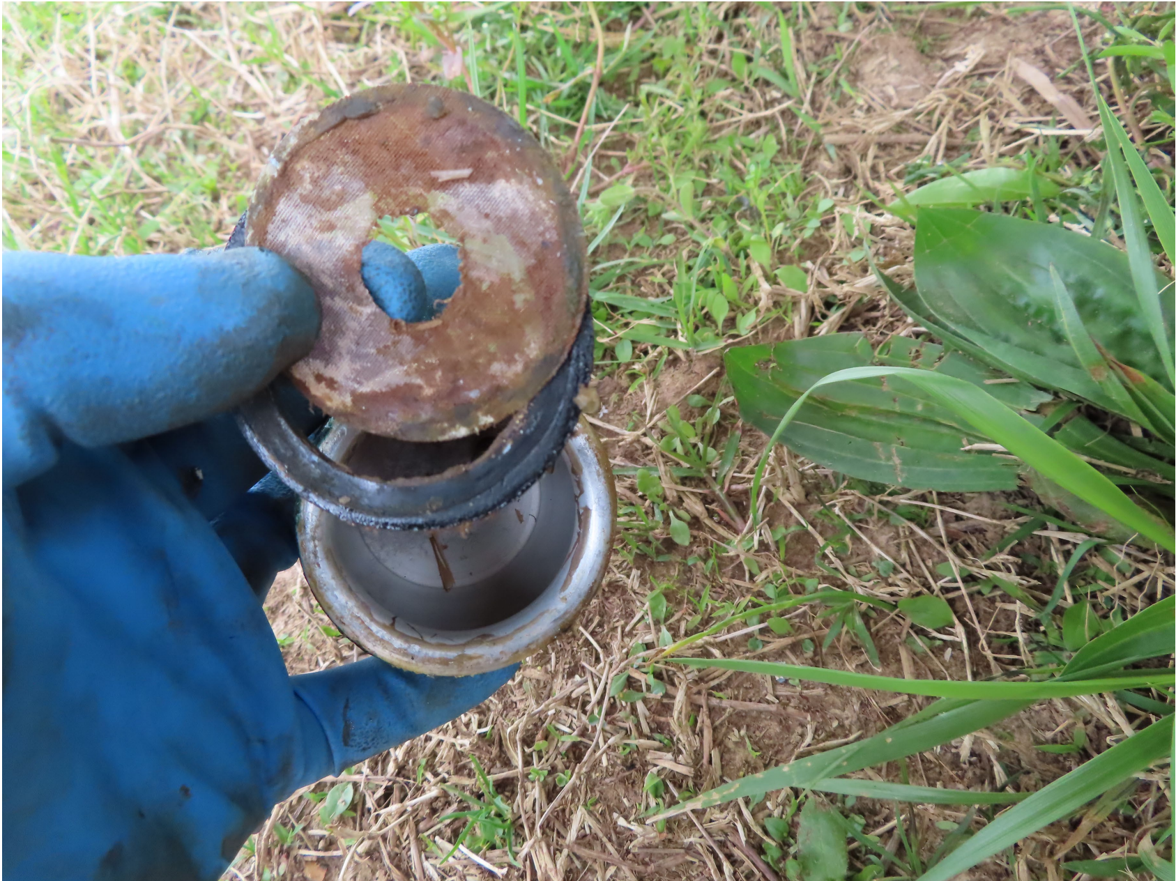
Photo 7 – Right Wing Gascolator with Occluded Debris Screen as Found (Piper)
