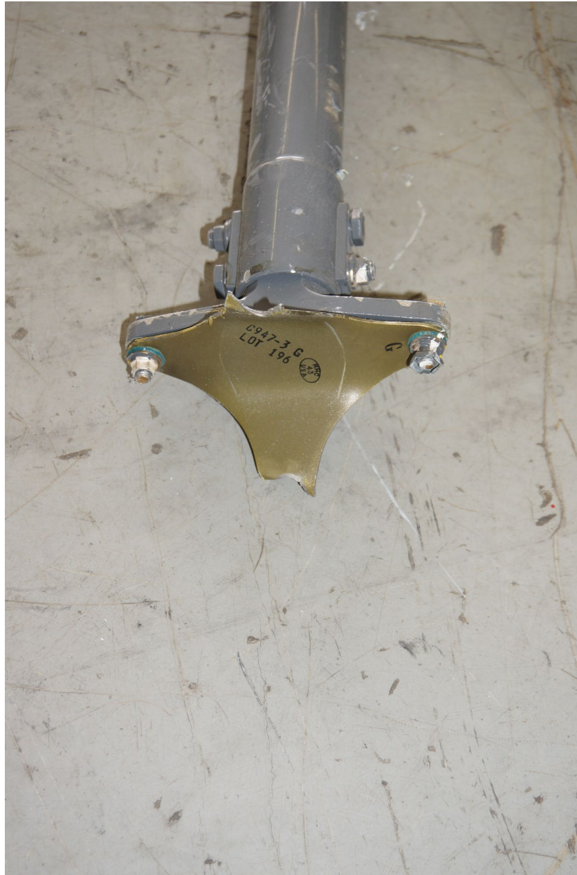
Photo 15 – Broken Flexible Drive Shaft Coupling
