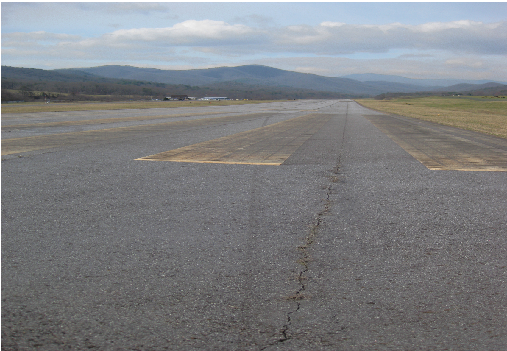
Photo 3 – View of runway looking west with airplane skid marks starting at 1,200 before runway end (FAA photo)
