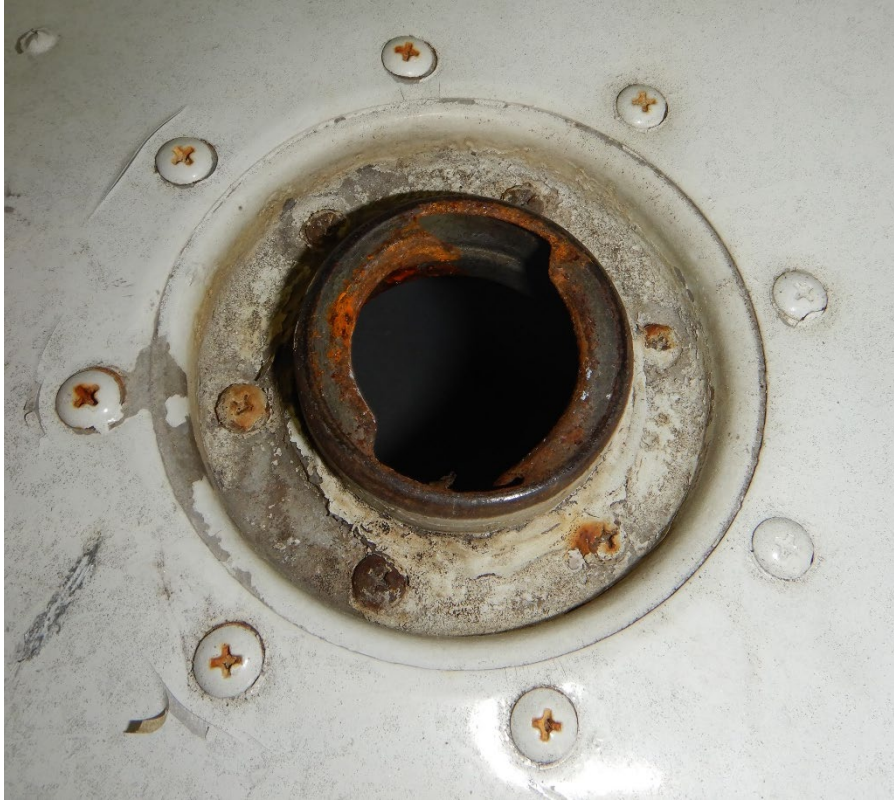
Figure 8: Right fuel filler neck exhibited corrosion
