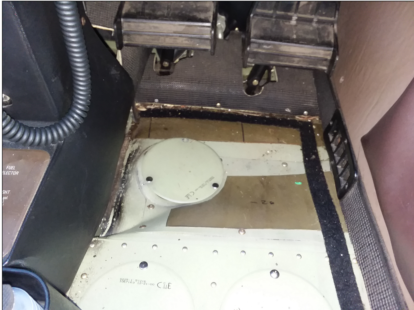
Photo 3 – Substantially damaged lower fuselage area located on right side of cockpit (Photo Courtesy of FAA)
