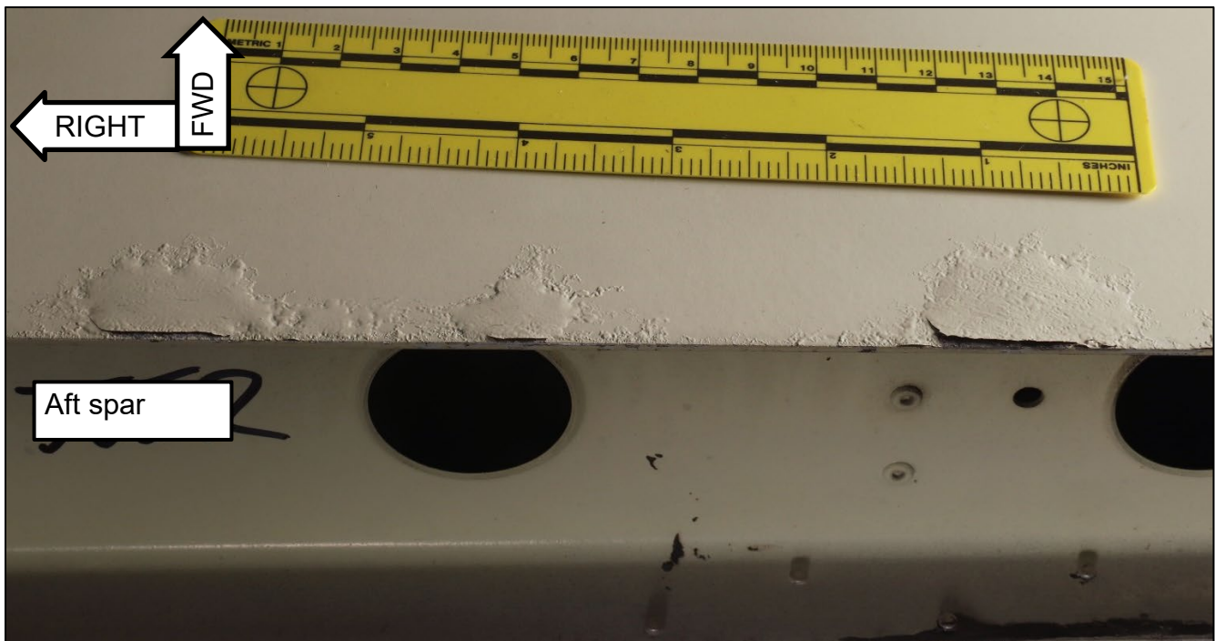
Figure 18. Trailing edge of the exemplar right horizontal stabilizer showing indications of corrosion with bubbled paint at the trailing edge of the lower skin near mid span.
