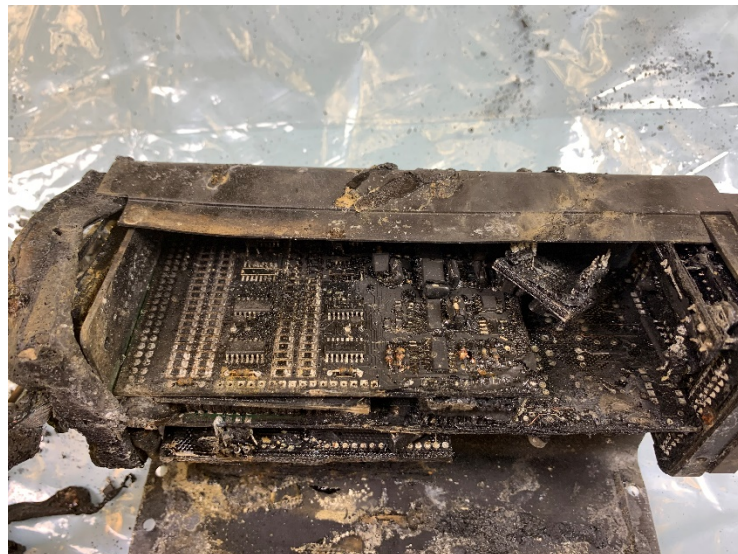
Figure 2. Damaged interior of EDM.
