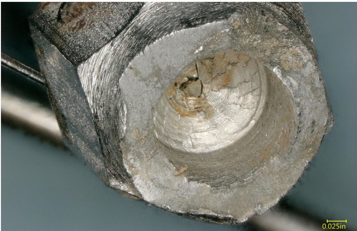
Figure 11 – View of the stud side (cockpit side) terminal stud fracture surface after second cleaning.
