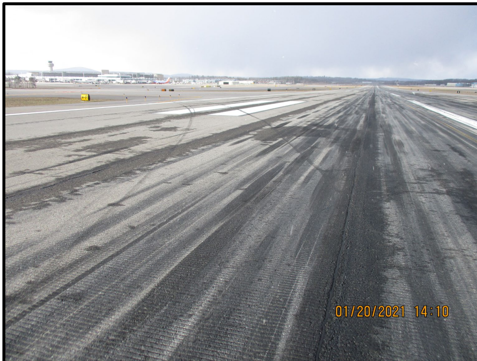
Figure 12-Tire skid marks on runway 35 from N641WA.
