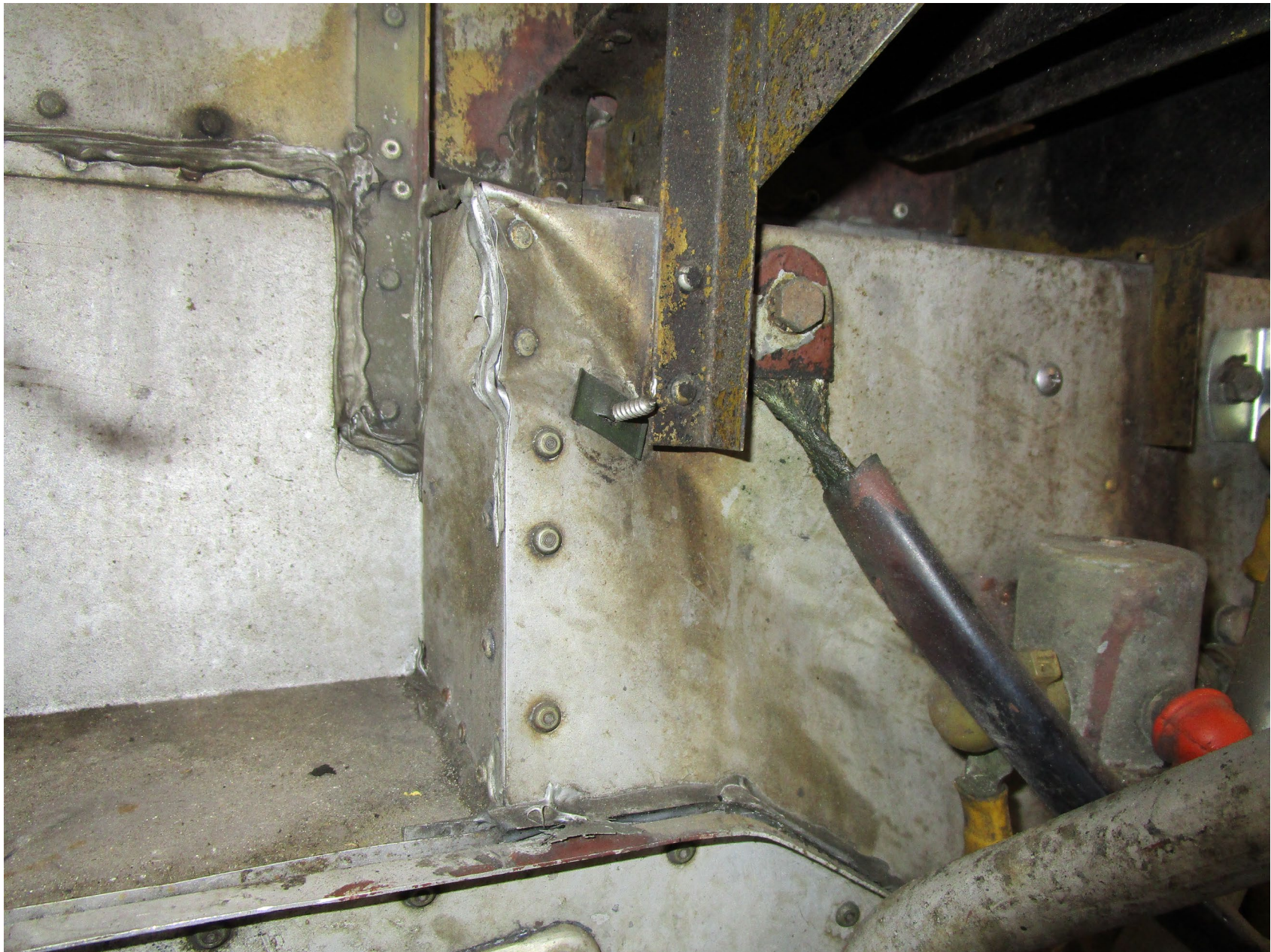
Photo 2 – Damage to Firewall (Provided by FAA)
