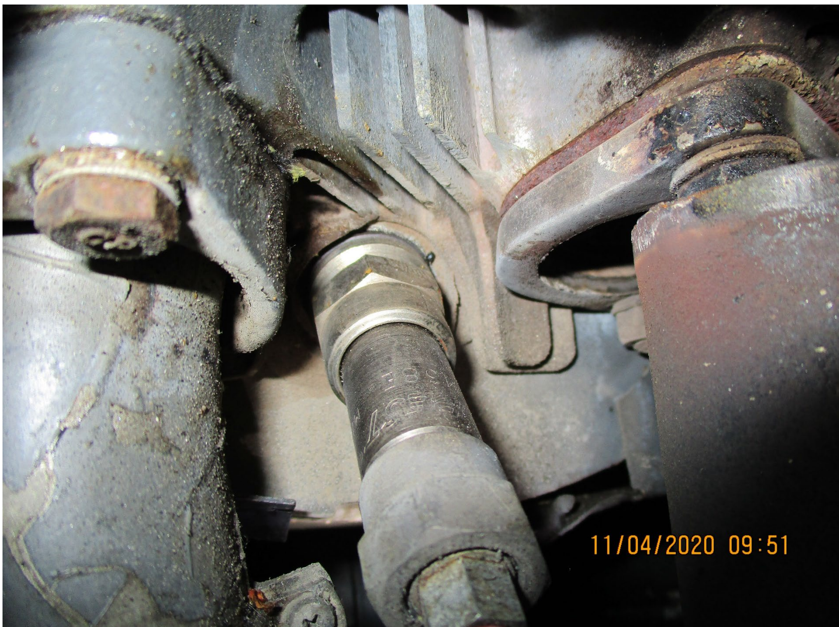
No. 2 Cylinder Soot on Exhaust Flange (IMG0168 - Photo Courtesy FAA)
