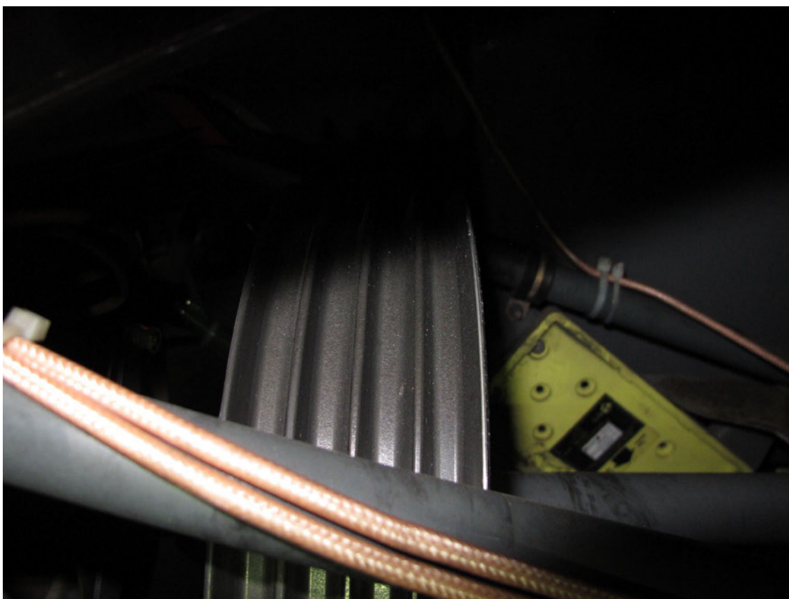
The upper sheave grooves.
