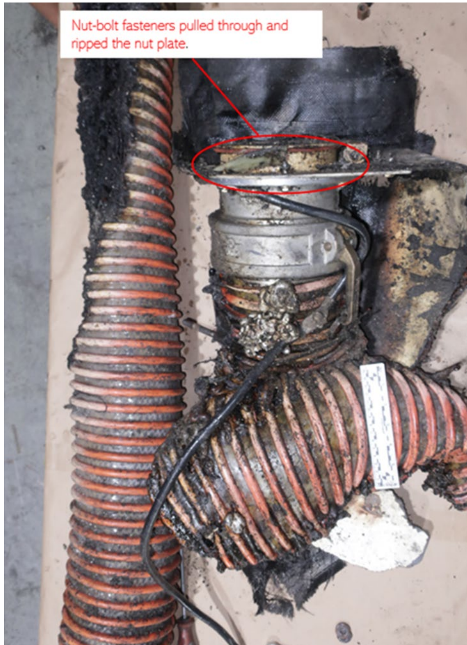
Figure 14. Aft side of the fire tank nozzle support and the snorkel hose connection.
