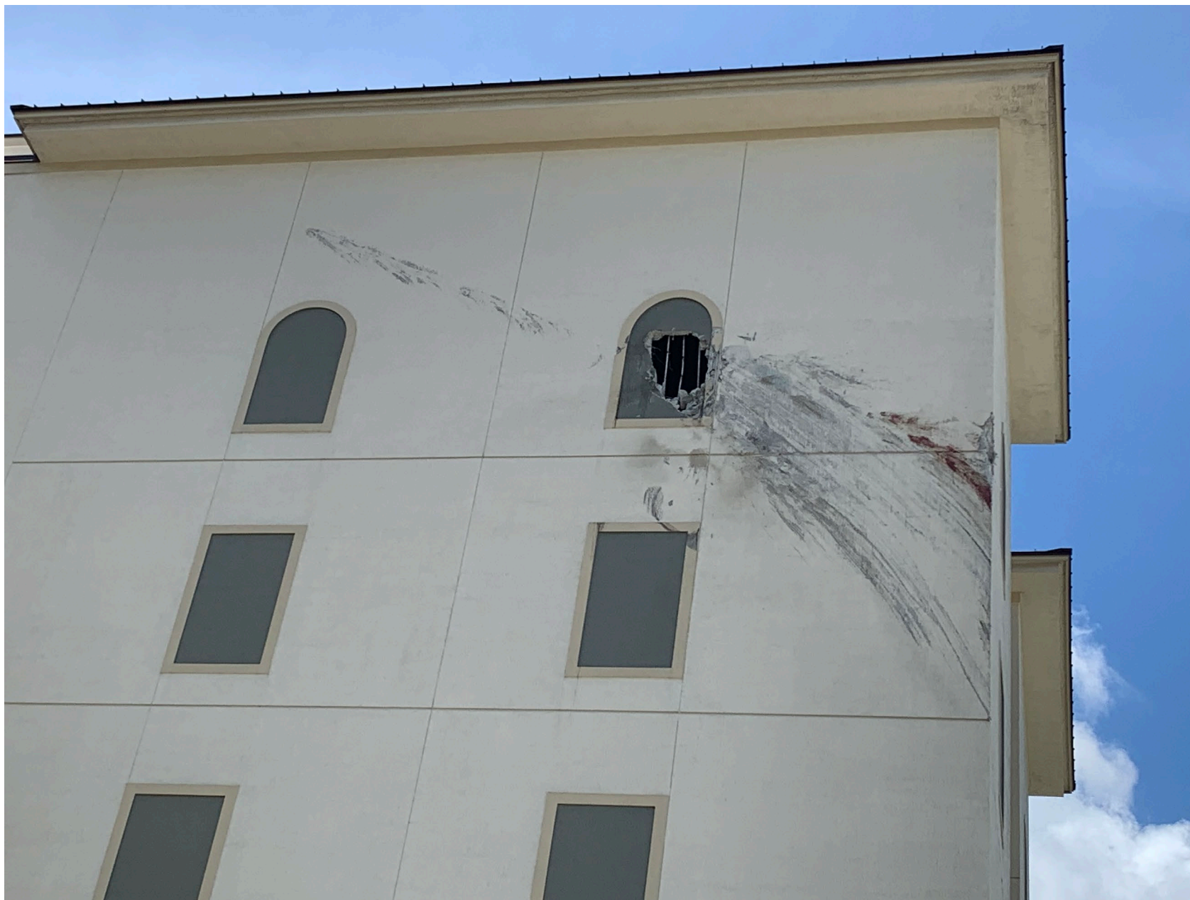
Photo 3 – FAA Digital Photograph. View Depicting the Building Impact Point.
