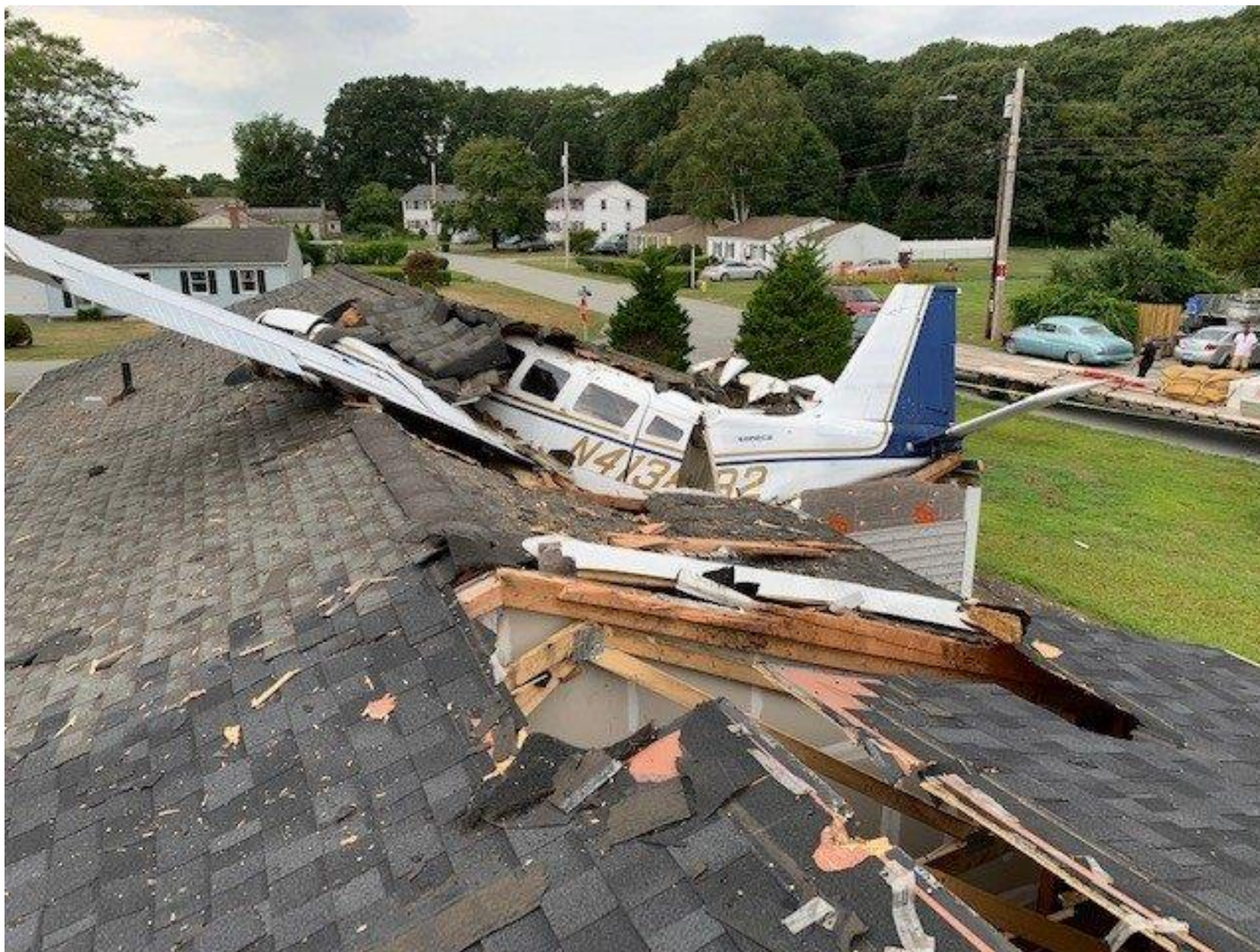
Photo 2 - Digital Photograph From Insurance Adjuster. View of the Airplane on the Roof Before Recovery.
