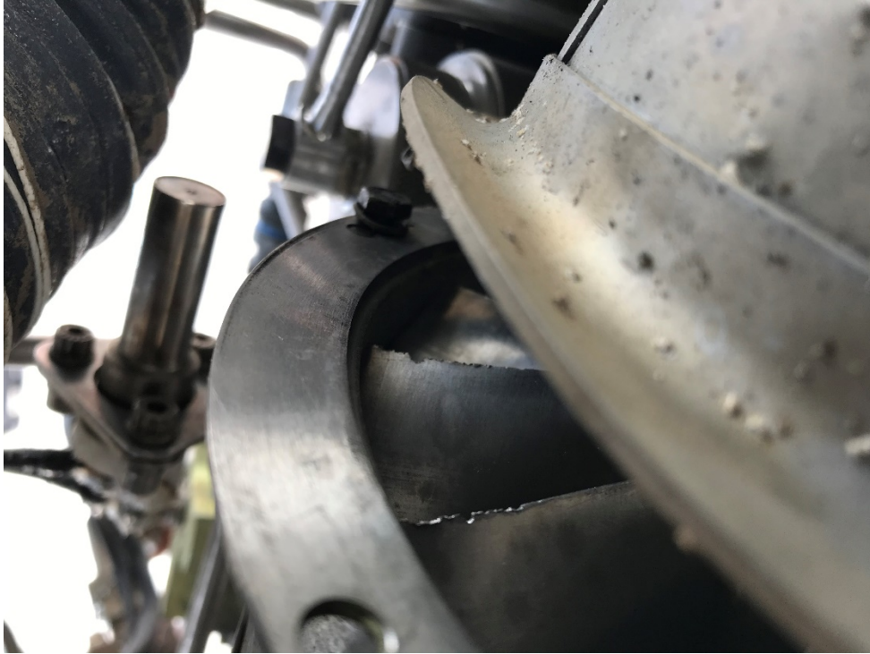
Photo 13: Axial compressor FOD damage
