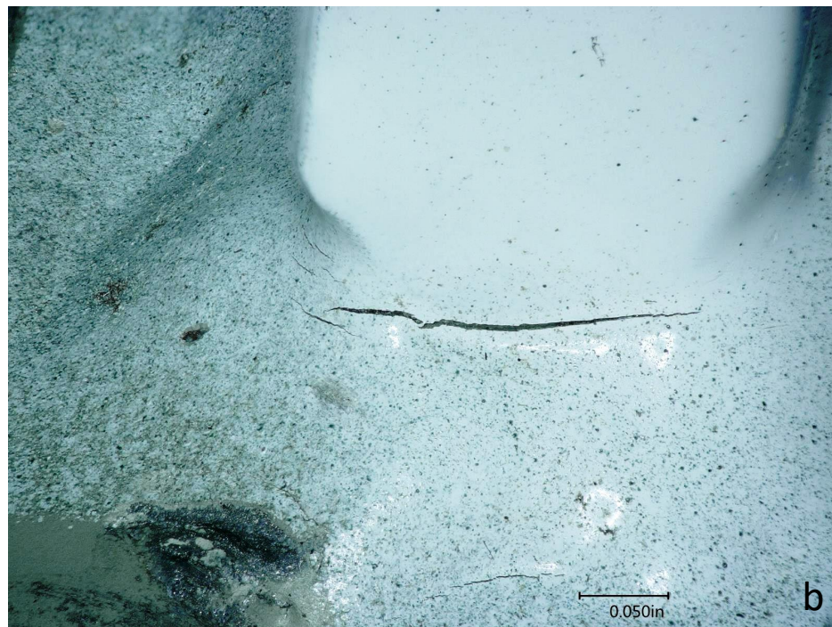
Figure 14 Views of the weld deposit between the upright and the base plate closest to bolt hole 3. Cracks in the paint film and disbonded paint are observed.
