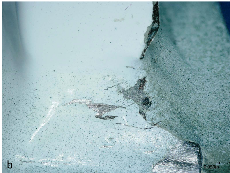
Figure 13 Views of the weld deposit between the upright and the base plate closest to bolt hole 2. Cracks in the paint film and disbonded paint are observed.
