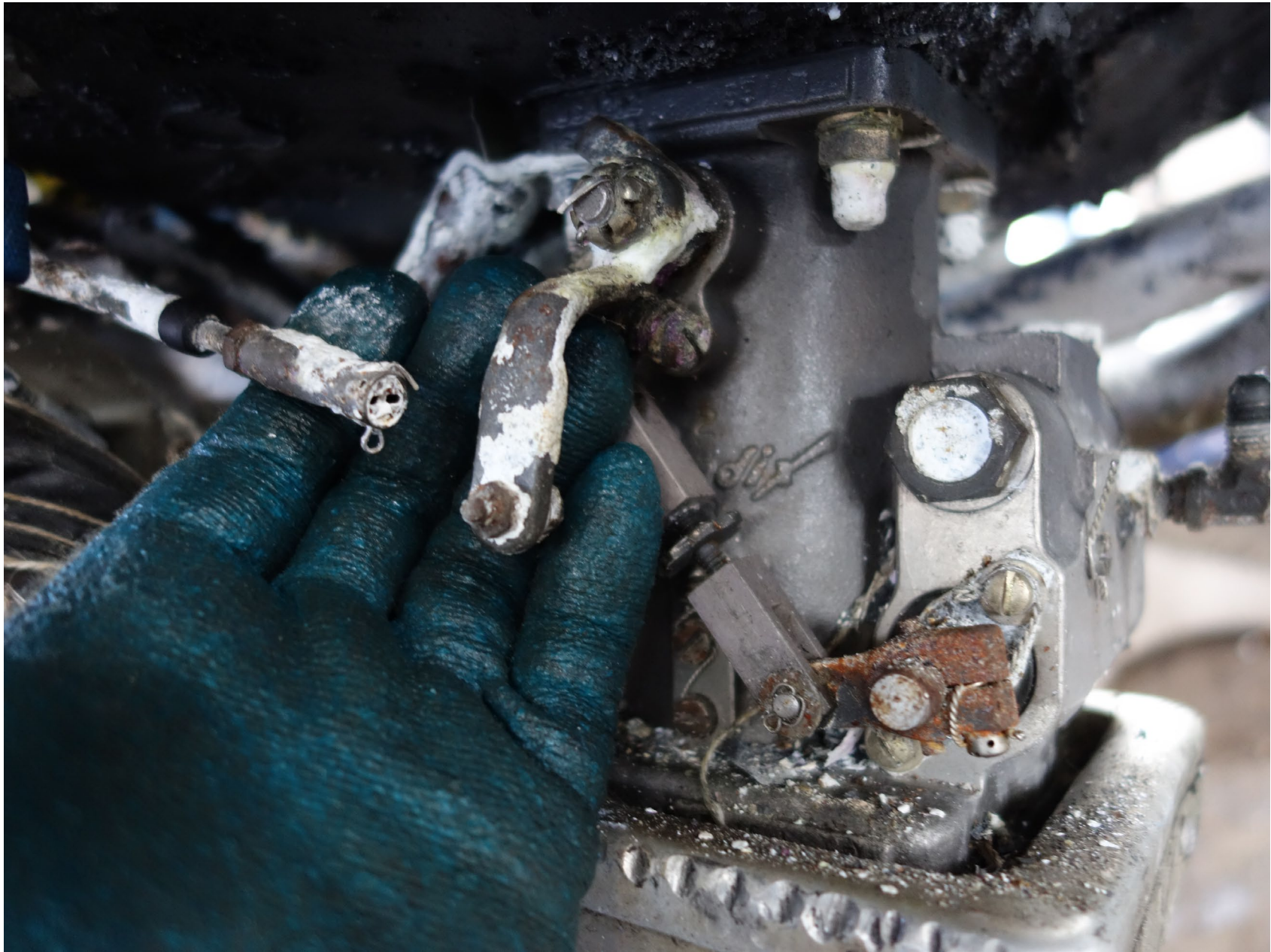
Photo 9 - Piper Digital Photograph. View Showing the Separated Throttle Control Cable at the Left Servo Fuel Injector.
