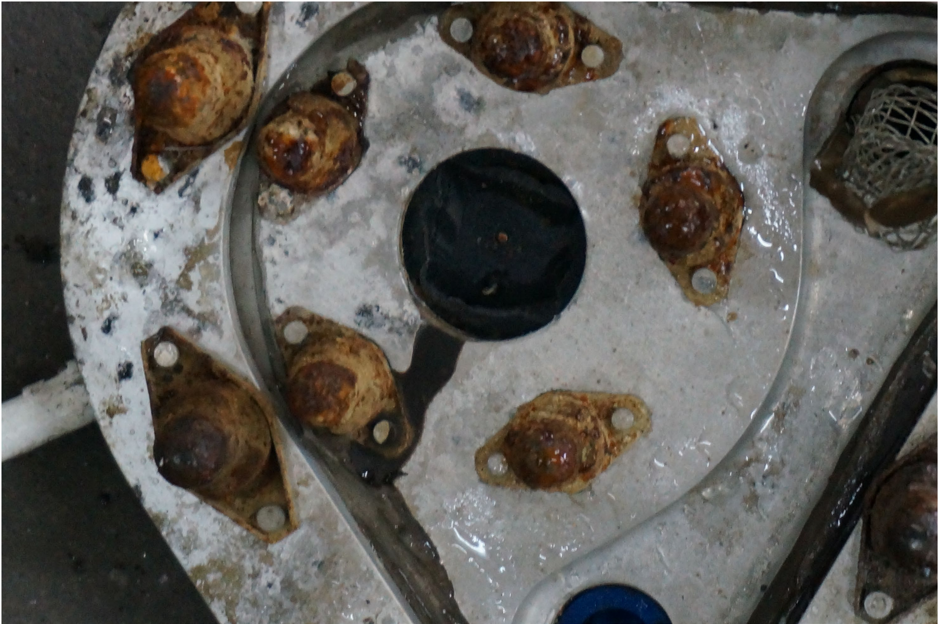
Photo 19 – Close Up of Fuel Tank Sump Flange (Probe Side)
