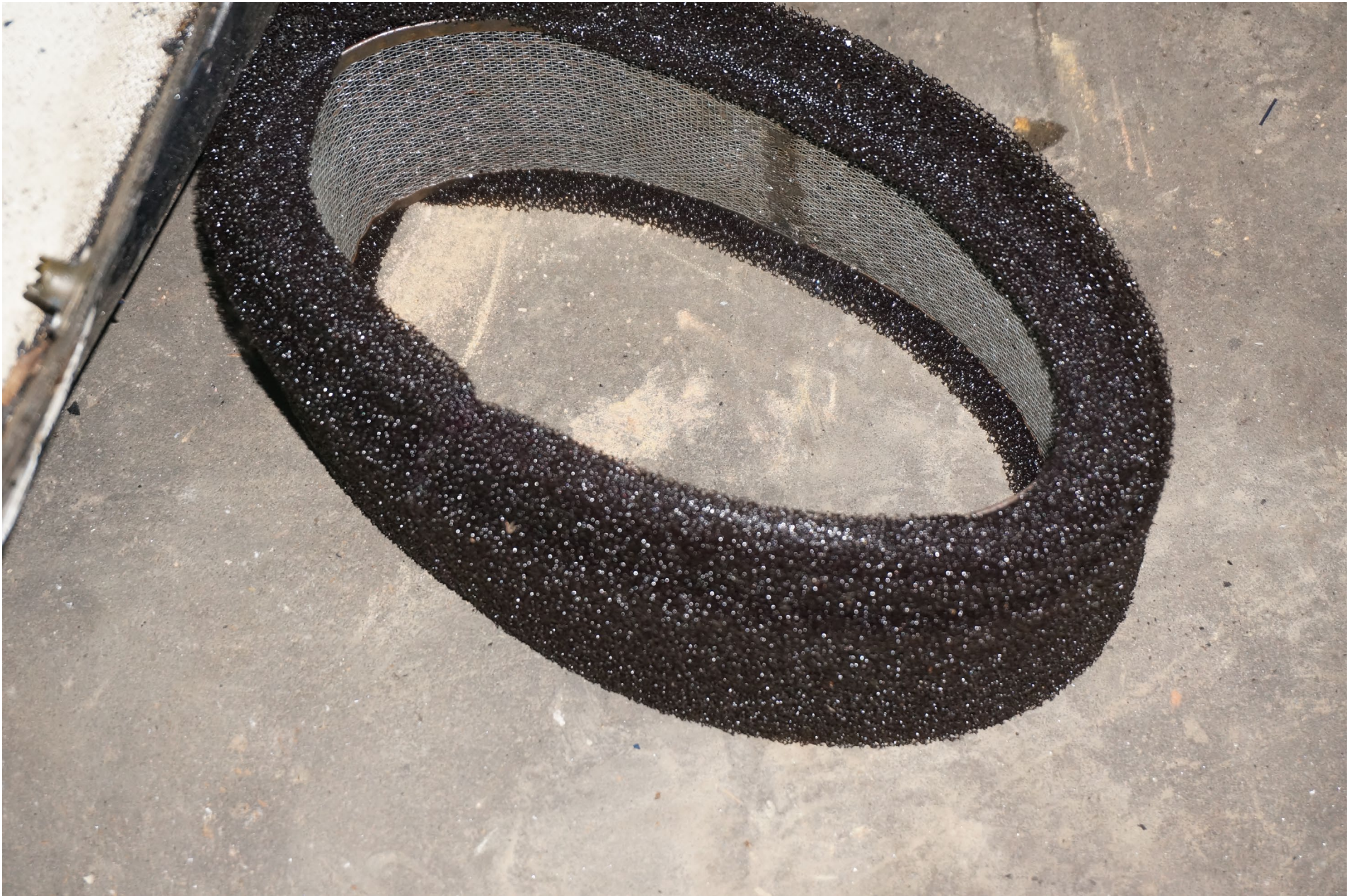
Photo 13 – Air Intake Filter
