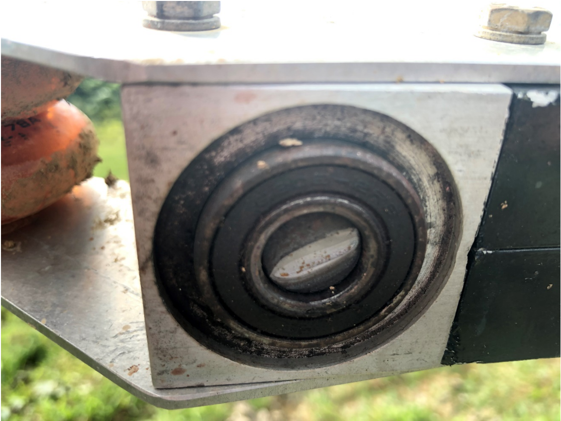
Figure 2. Closer view of fractured bolt.
