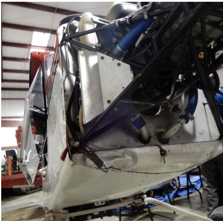
Figure 6. View of underside of airframe. Note: No oil streaks.
