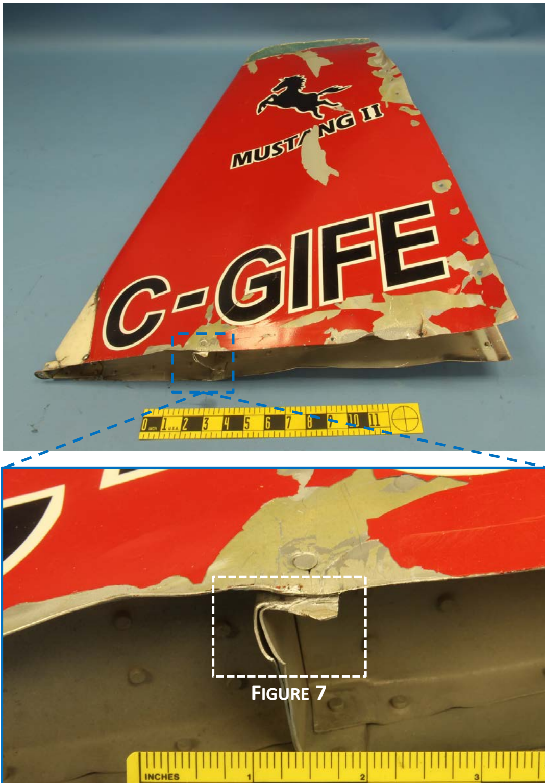
Figure 6: The top shows an overall photo of the separated vertical stabilizer. The bottom photo is a close-up of the left corner of the main rib doubler.
