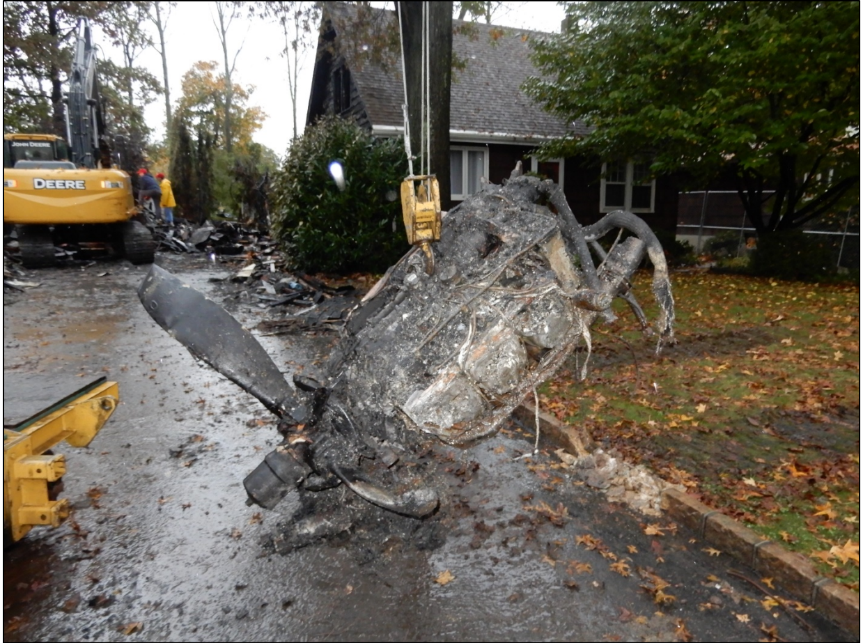
Photo 12: View of left engine being hoisted away from the housing debris.
