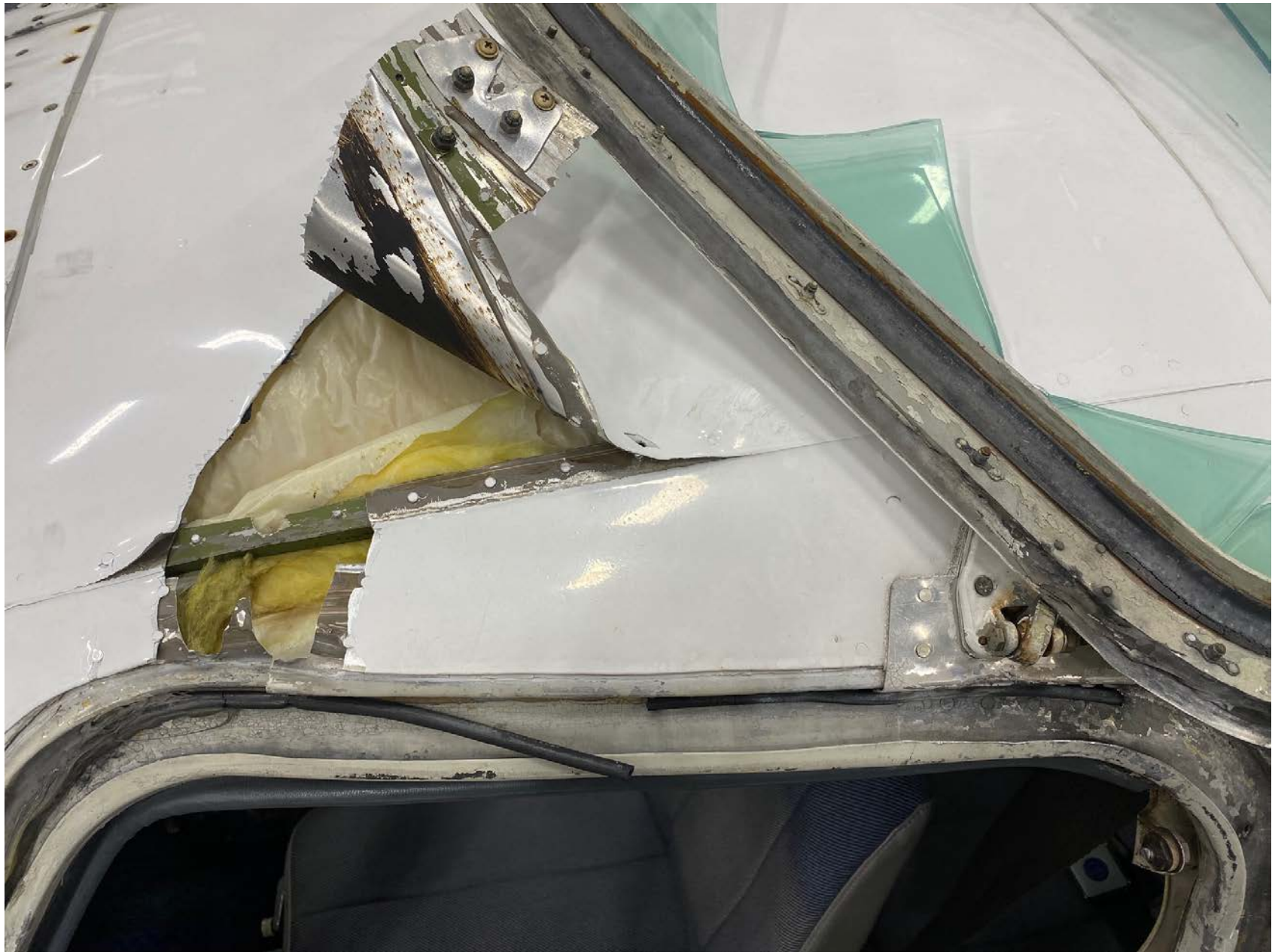
Photo 2 – Close-up View of Damaged Structure (Cape Air)
