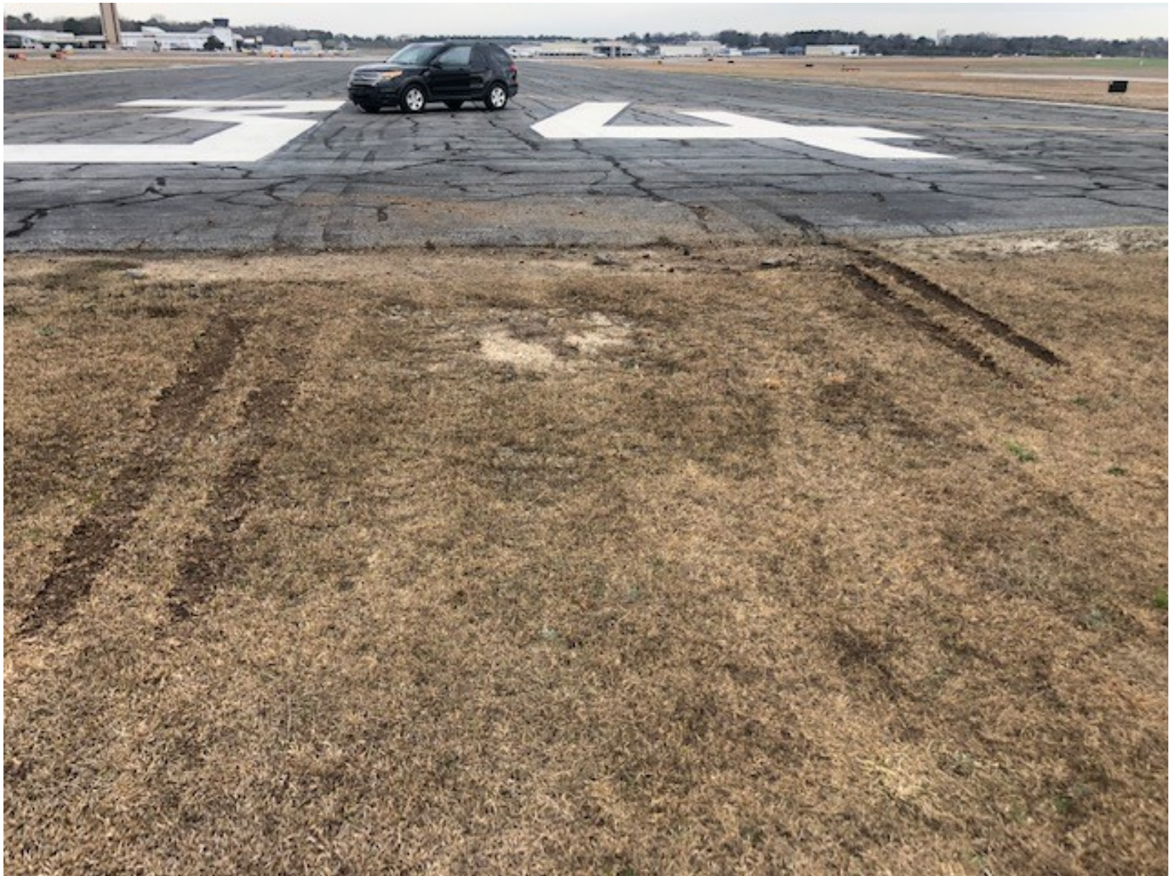
Photo 3 – View of Airplane Tire Tracks and Runway 34 (Photo Courtesy of FAA)
