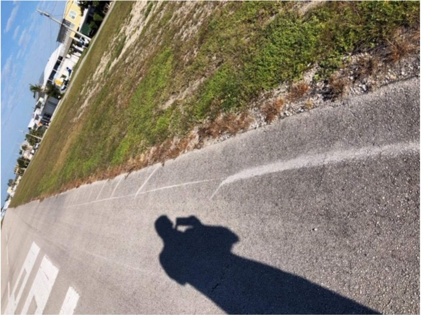
Photo 1 – Runway Scrape Marks (Photo Courtesy of FAA)
