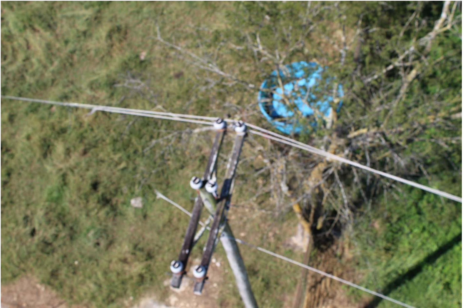
Photo 14 – Damaged Power Lines (FAA Photo)
