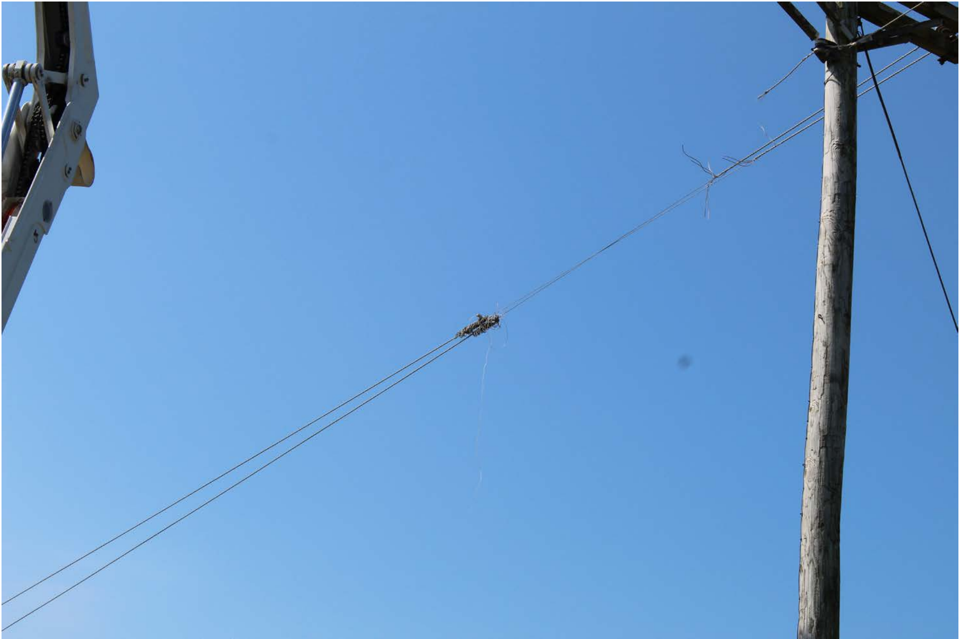
Photo 13 – Damaged Power Lines (FAA Photo)
