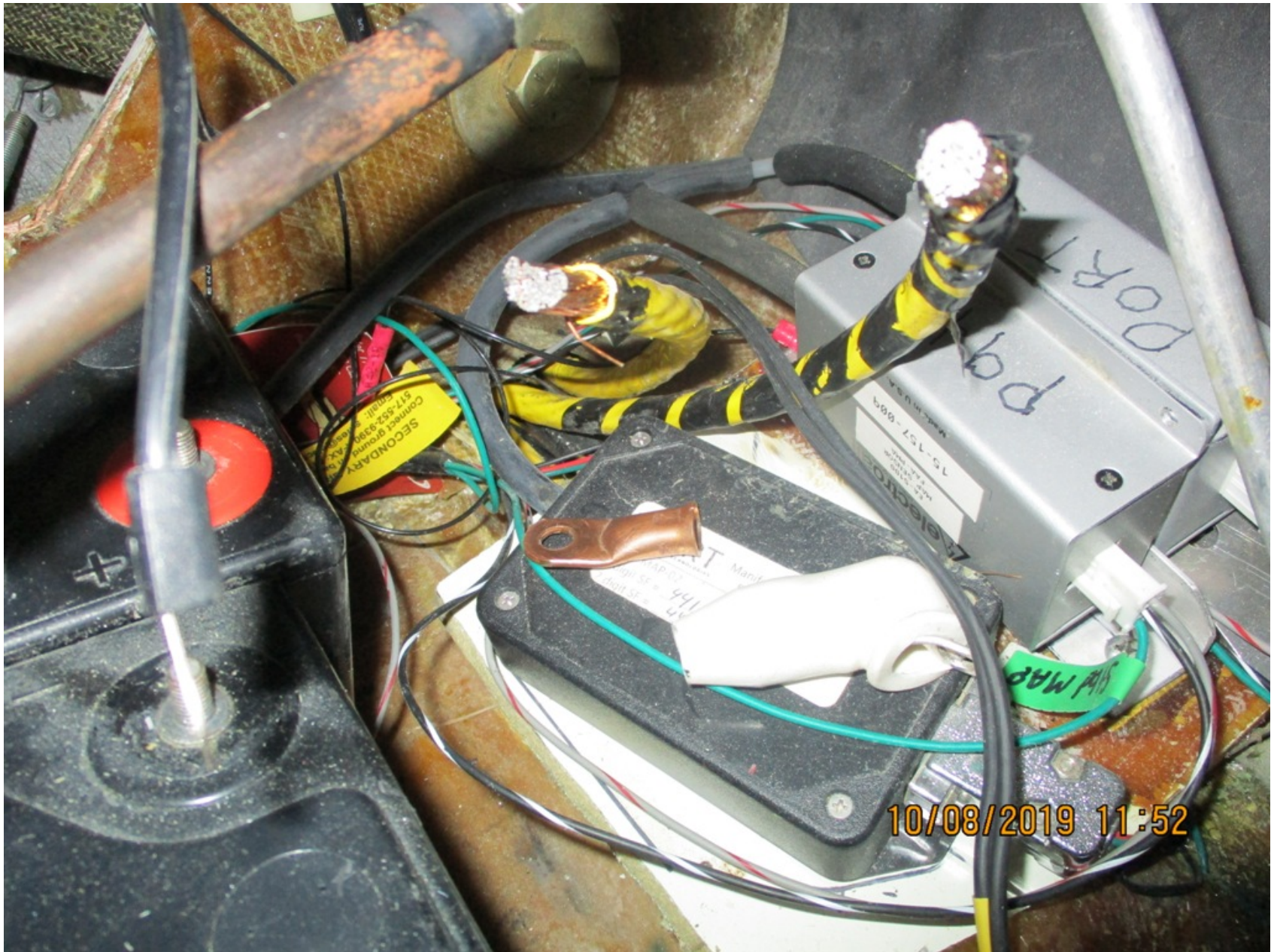
Photo 3 – 24v Battery Negative (left) and Positive (right) Leads (photo NTSB)
