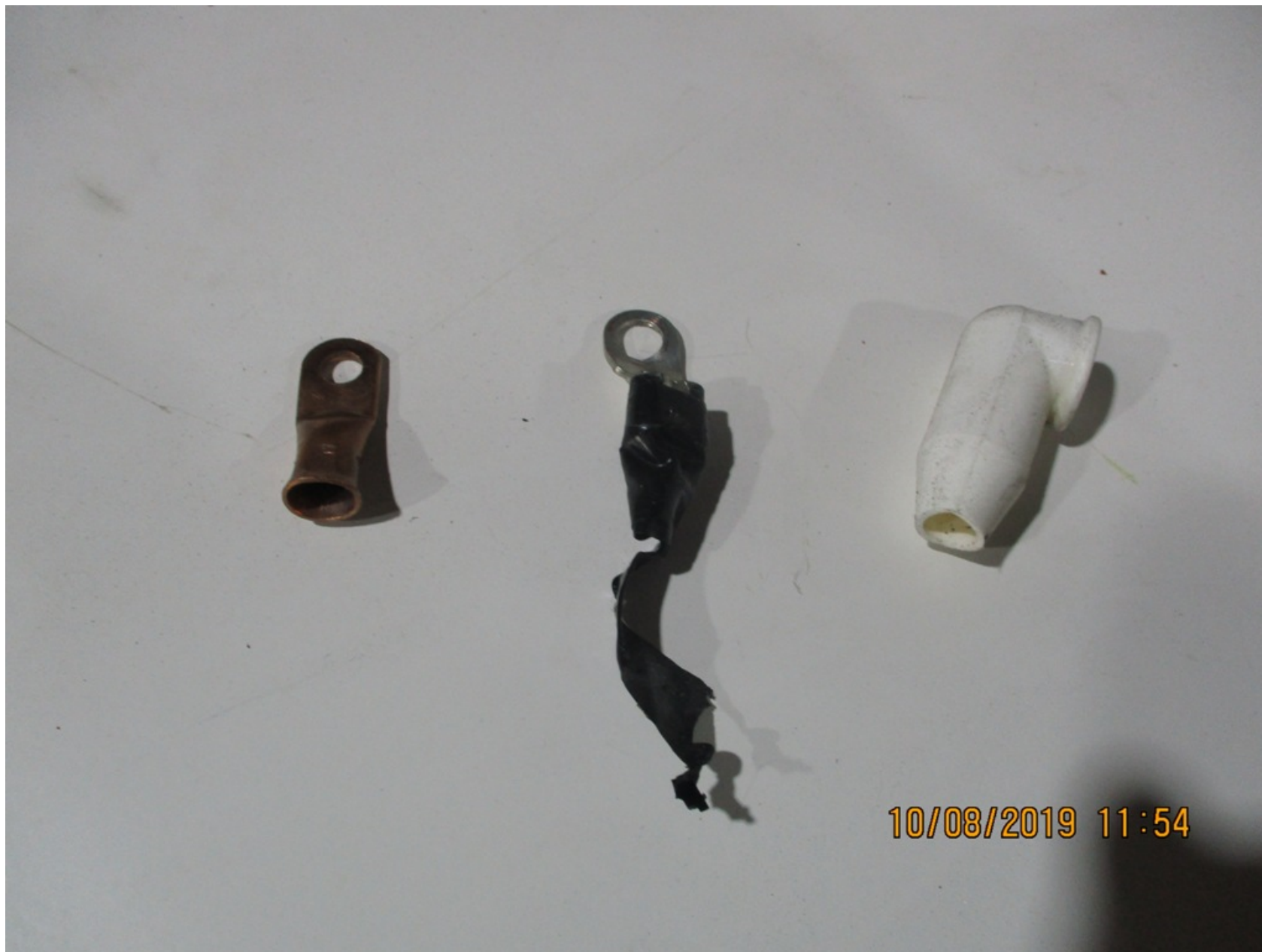
Photo 4 – 24v Positive (left) and Negative (right) Battery Connectors (photo NTSB)
