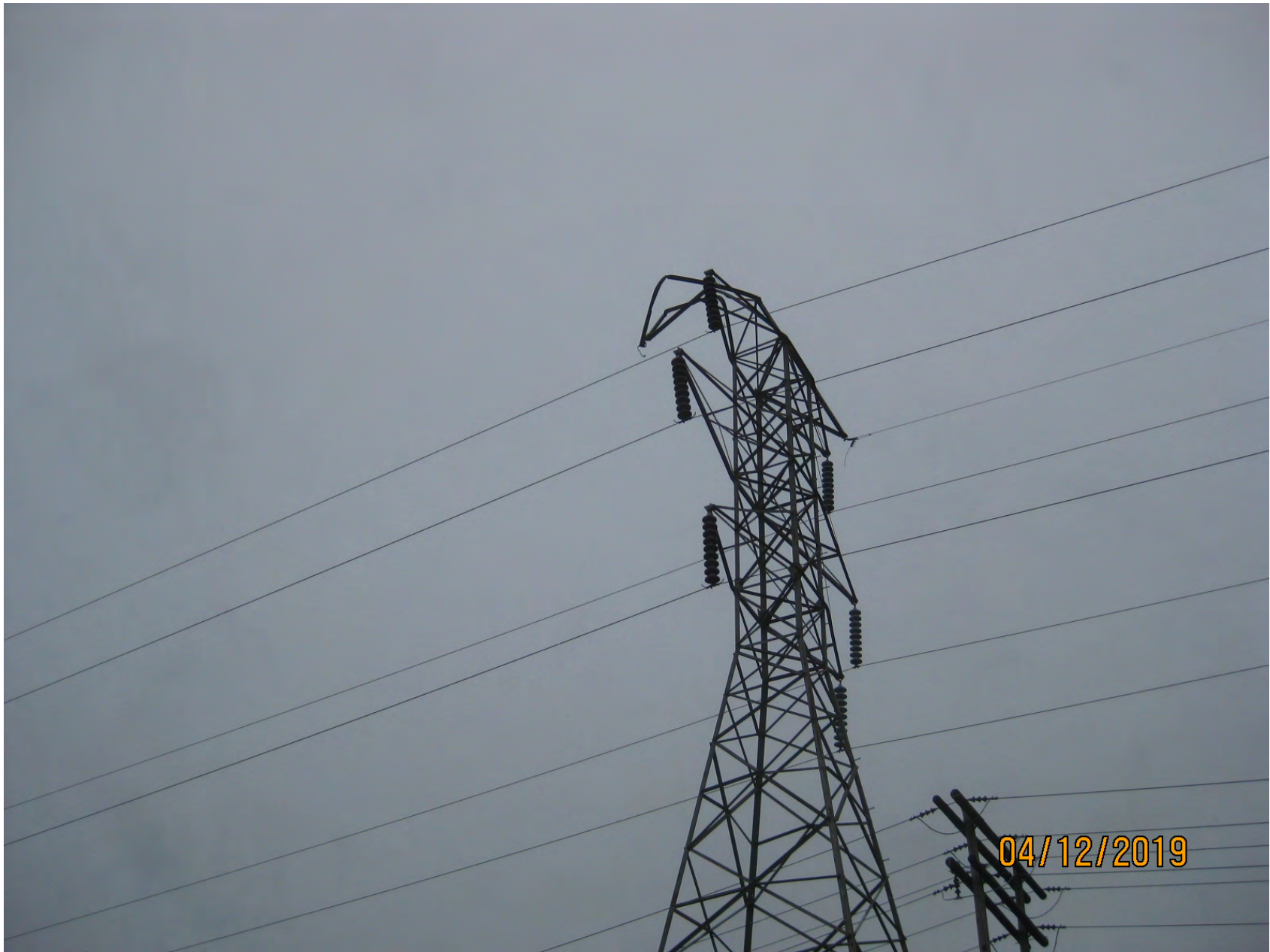
Photo 8 – Damage to power lines (Photo courtesy of FAA)
