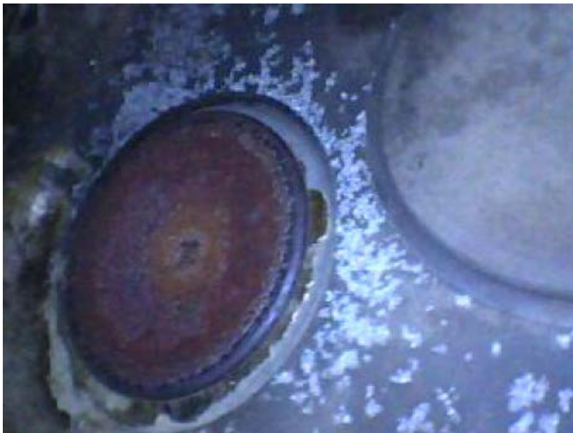
Figure 7: No. 1 cylinder valves
