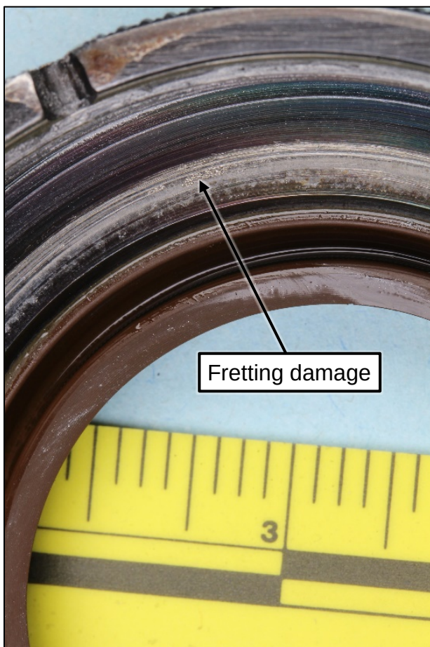
Figure 13. Fretting contact damage on the interior face of the bearing retainer nut.
