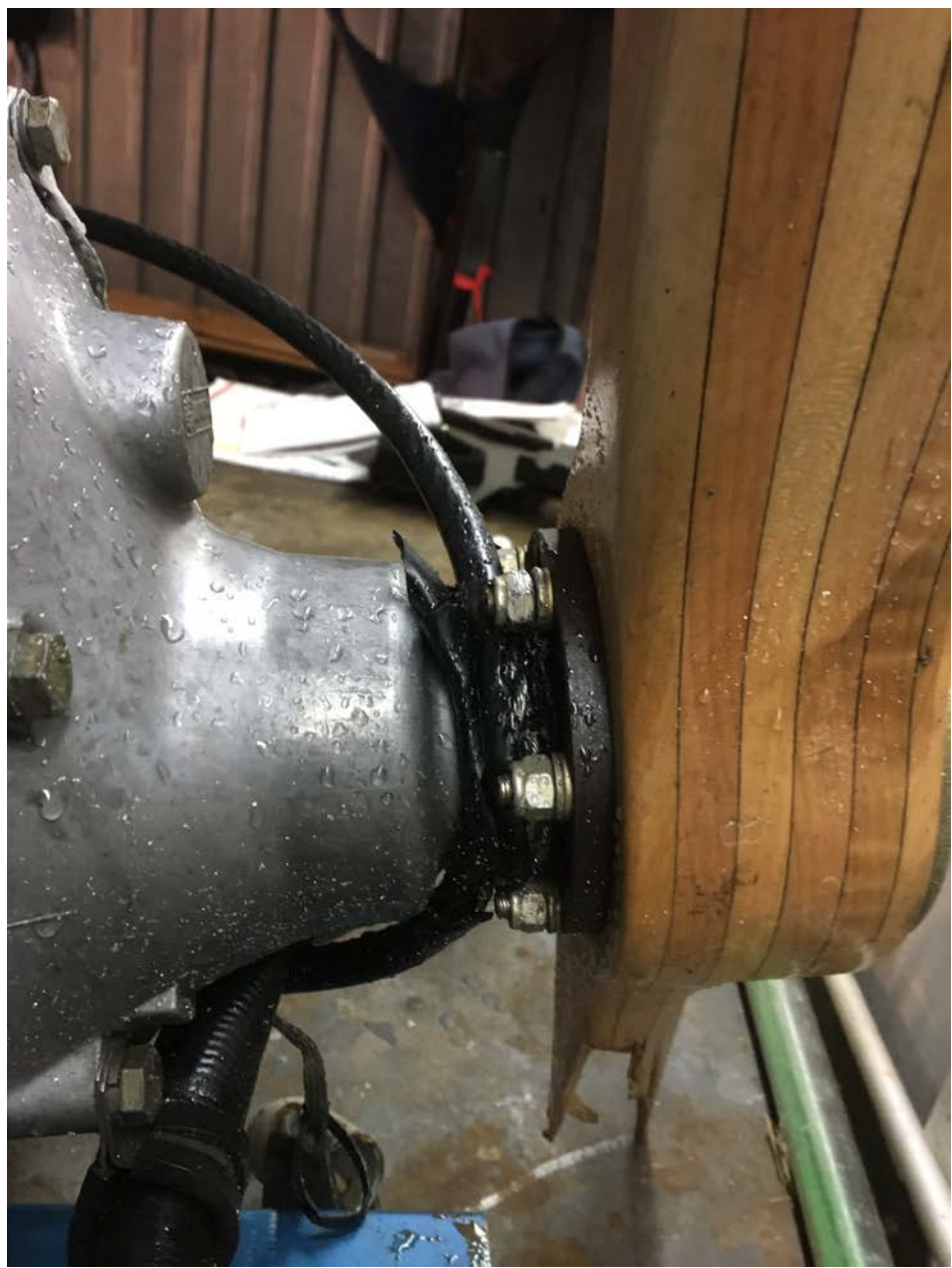
Photo 5 – View of BRS Cable Wrapped around Propeller Hub
