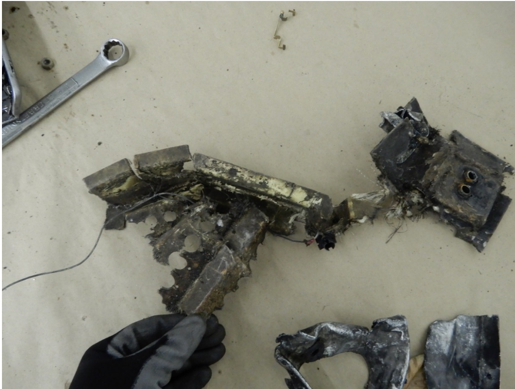
Remnants of circuit breaker panel, NTSB photo
