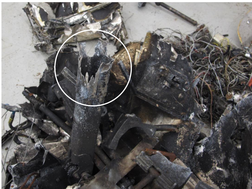
Figure 5. Thermal tearing of pedestal (highlighted in white circle).
