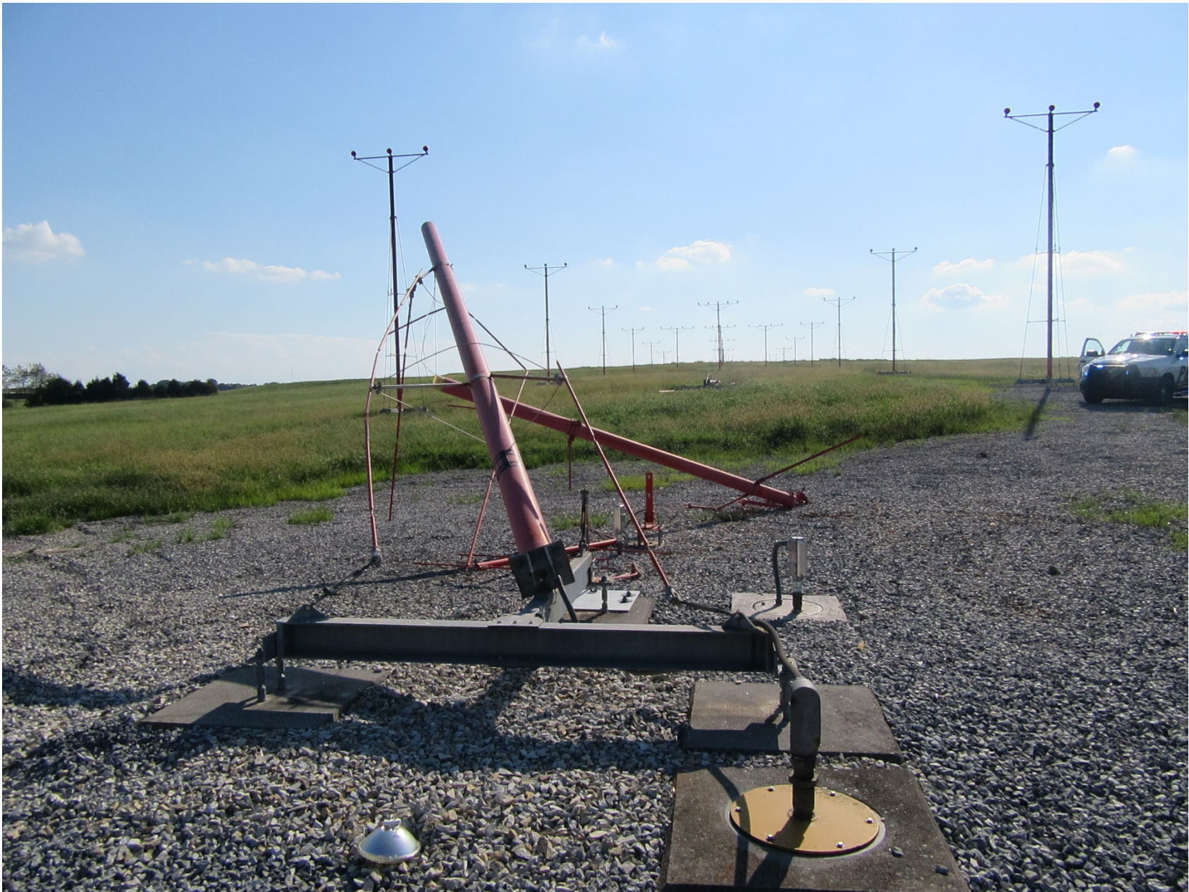
Photo 3 – View of Damaged Approach Lights (Photo Courtesy of FAA)
