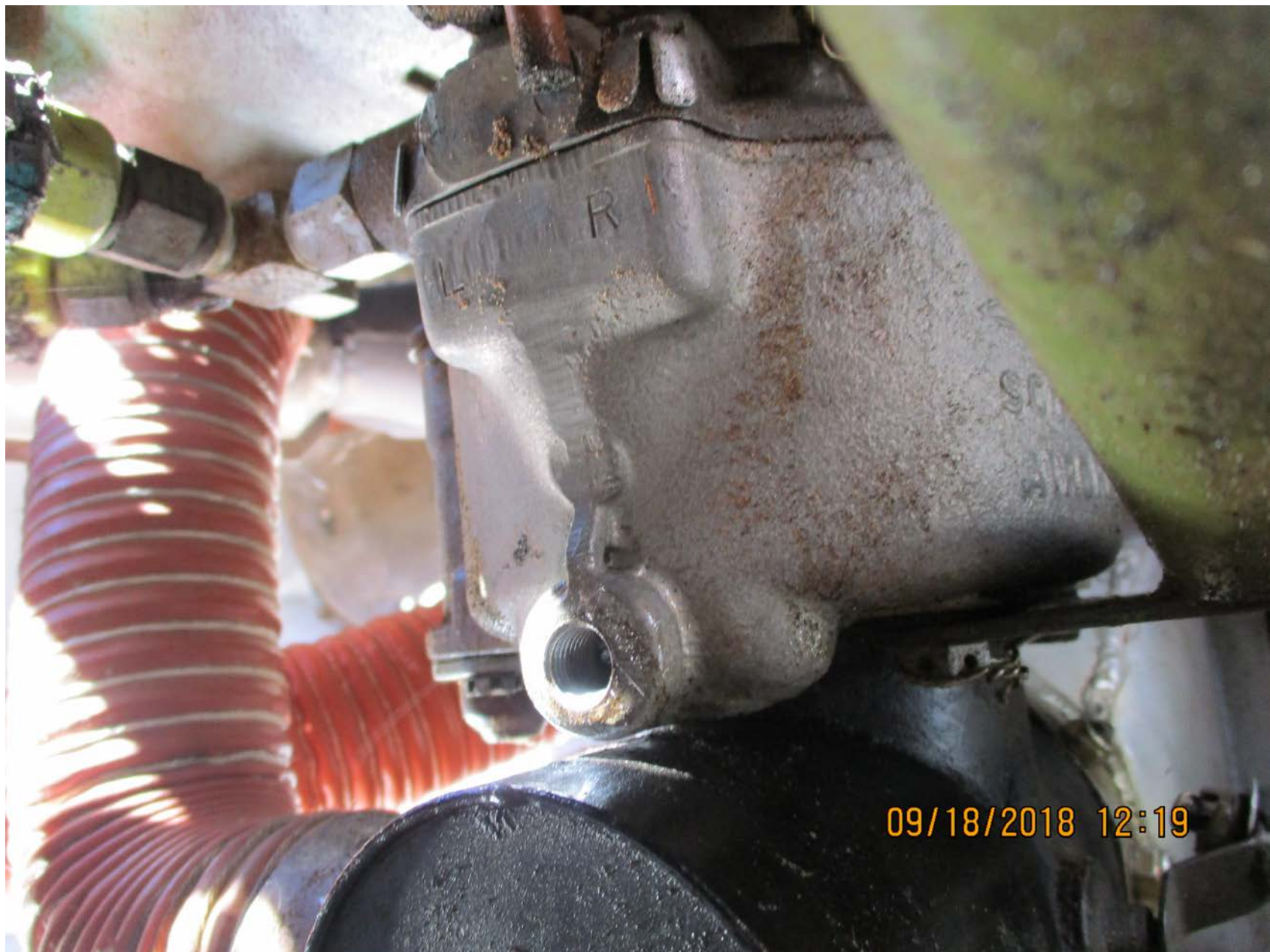
Photo 4 – Carburetor, plug missing
