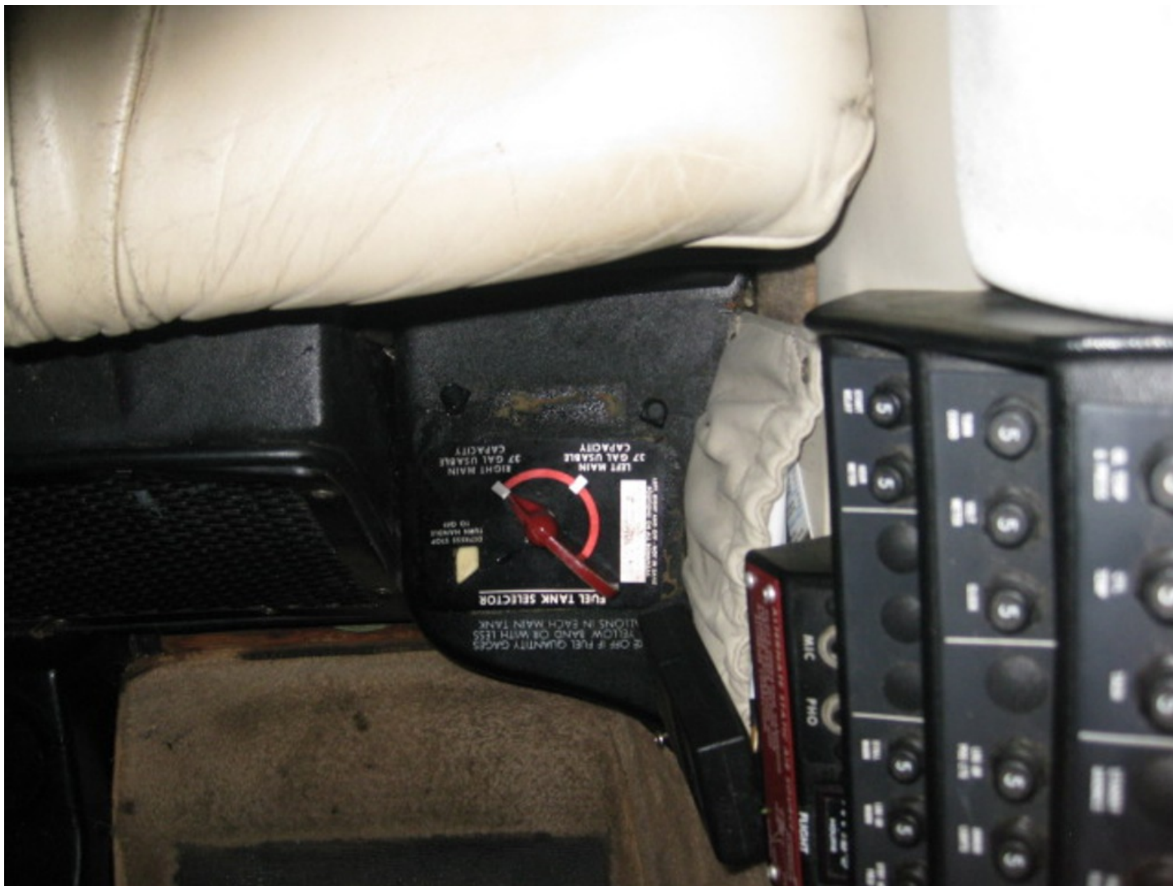
Photo 5 - FAA Digital Photograph. View of the Fuel Selector Valve in the Right Main Tank Position.
