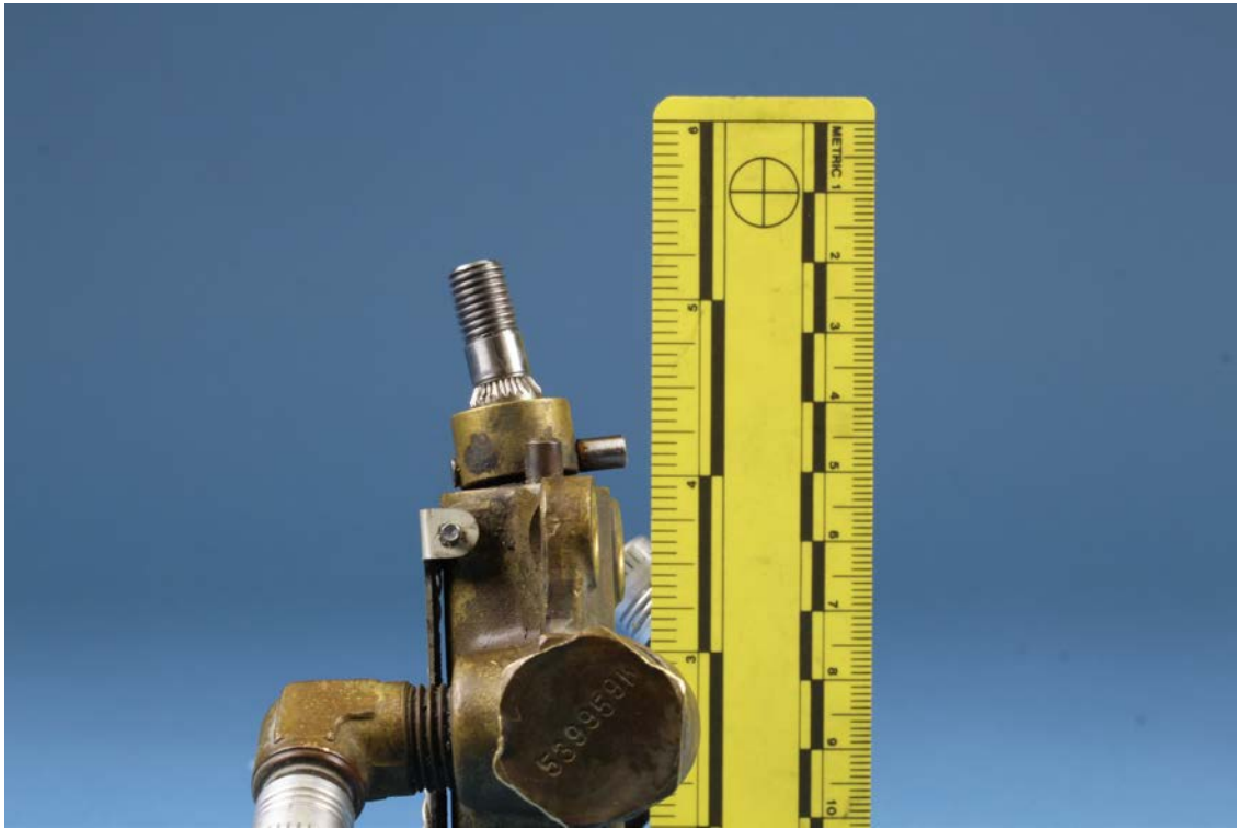
Figure 2: Bent control stem on metered fuel assembly.
